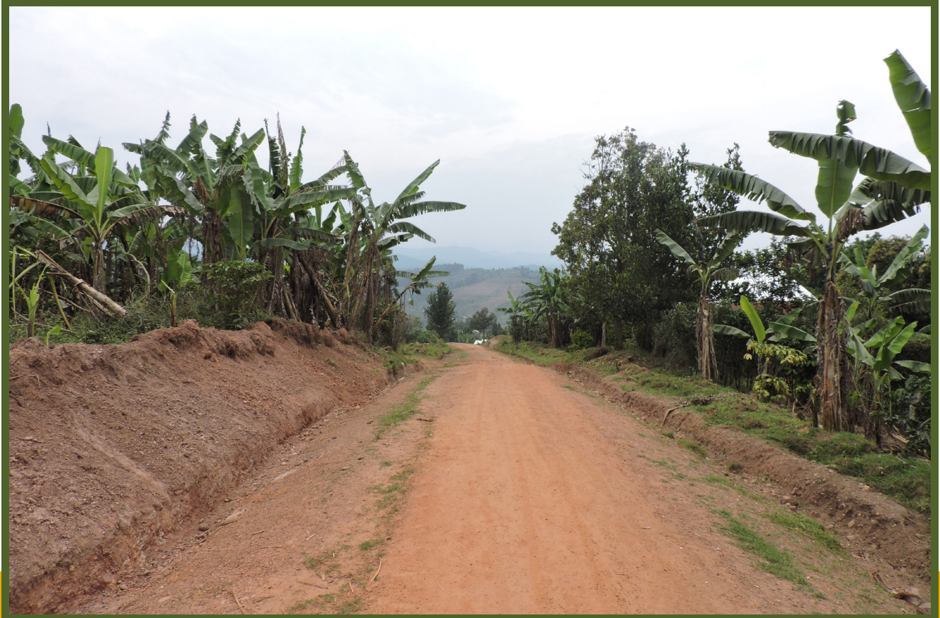
Plate 8: A road connecting Rubimbwa and Rutugunda Parishes in Kirima S/C, Kanungu District supported under TRS
