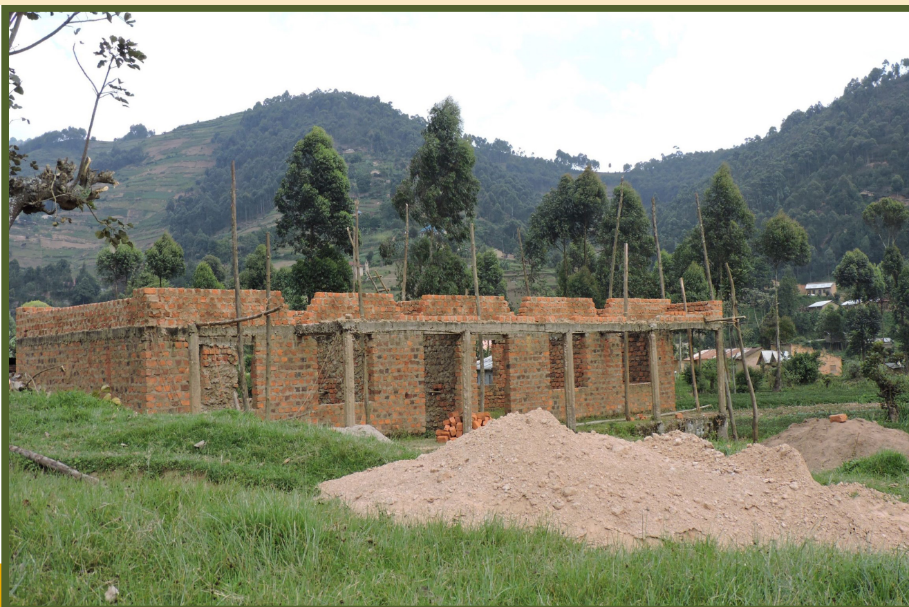
Plate 3: Construction of a 2-classroom block at Ndego S.S, Kashasha, Ikumba, Rubanda District (FY2018/19-2021/22)
