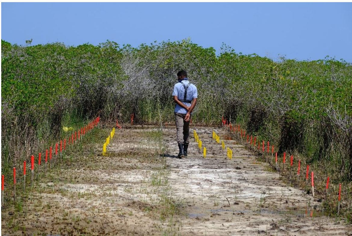
A manually cleared breach lane through mangrove trees on the edge of Maruthenkerny Lagoon: yellow marking sticks indicate the position of mines that have been found and removed, and red sticks indicate the boundary between safe and unsafe land. Photo courtesy of E. Chrystie
