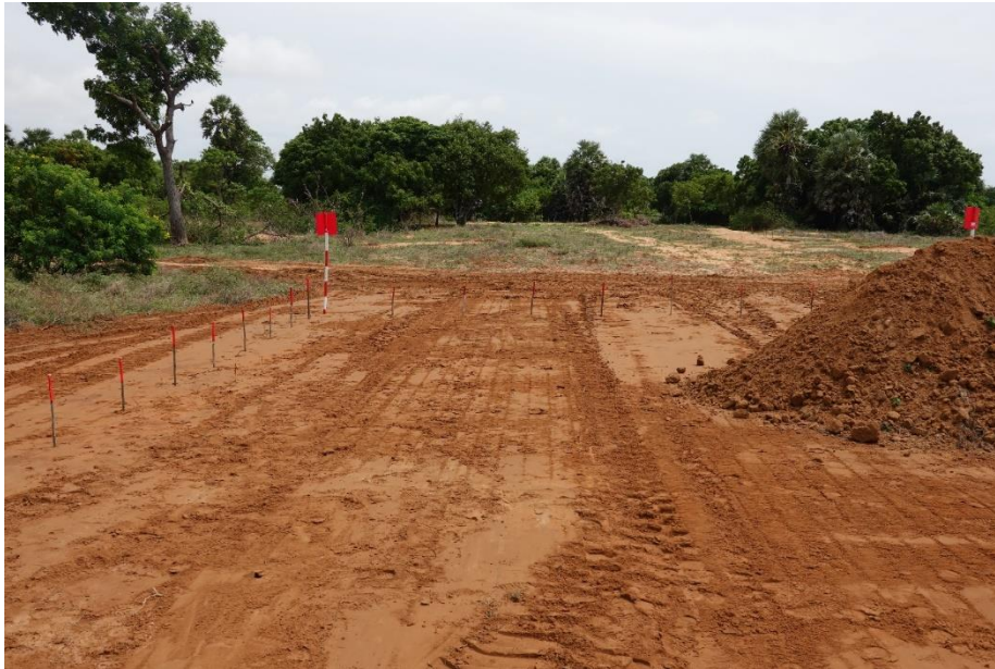
An area of mechanically excavated contaminated soil piled up and marked for follow on processing. Photo courtesy of E. Chrystie
